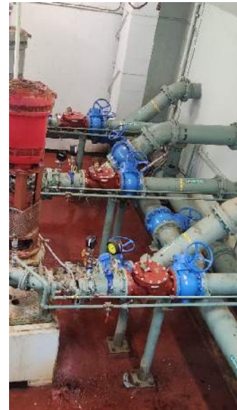
New plug and check valves installed at Bahia Main Pump Station.
