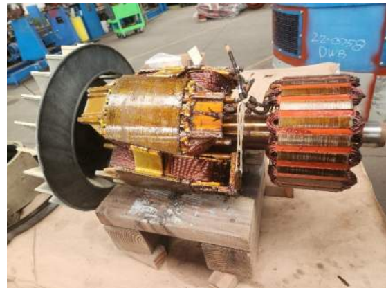
The Exciter Rotor and Stator being rehabilitated for the Meadow Park Standby Generator.
