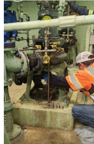
CSW II Eric Andersen removing rags from pump #2 at East Hamilton Pump Station
