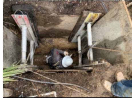
Figure 1: Broken VCP line being repaired by a contractor in an easement behind Peach Street.
