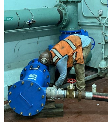
Figure 1: Bahia Main Ps Force Main condition assessment.
